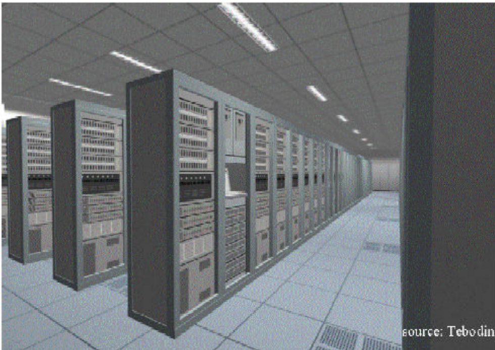
Figure 3-1: The “internals” of a data centre (Hartkamp, 2002)
